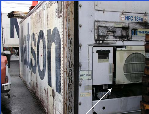
Simple banana ripening in a refrigerated Matson container in Hilo, Hawaii. Capacity: 320 boxes of bananas.
