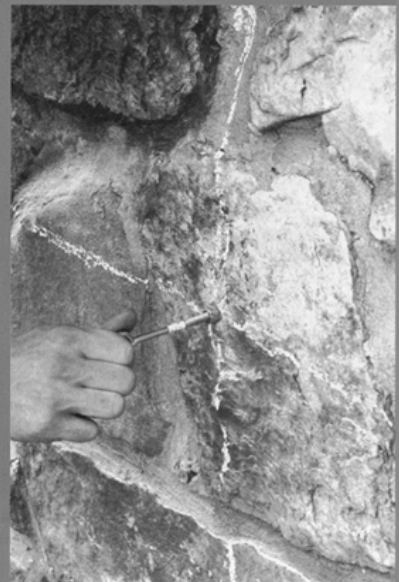
Screw eyebolts into the lag shields. The lag shields expand as the bolts are screwed in.
