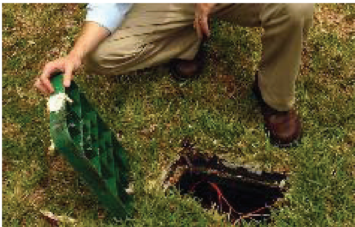
Figure 2. Open water meter. Credits: undefined
