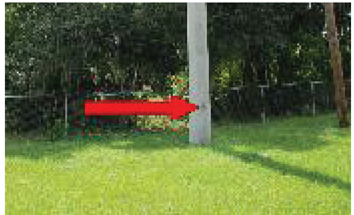
Figure 17. Small hole in power pole. Credits: undefined
