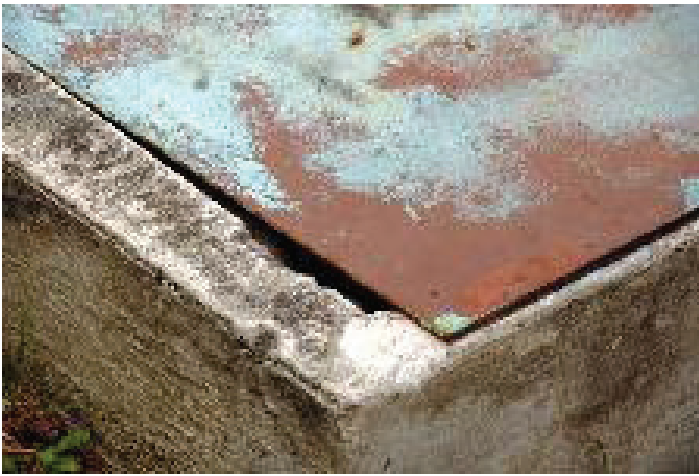
Figure 6. Crack in cement that creates opening. Credits: undefined
