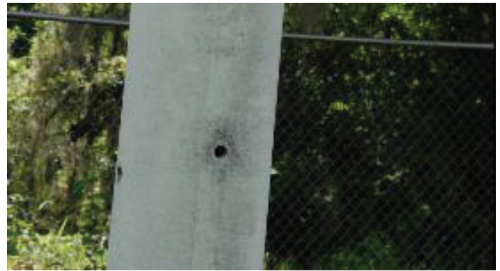
Figure 16. Small hole in power pole. Credits: undefined
