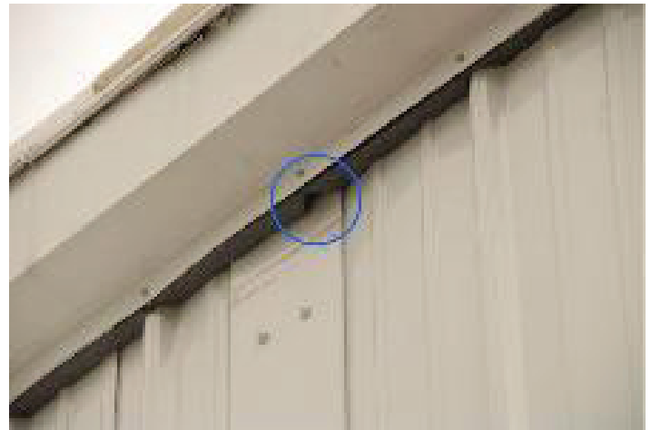
Figure 3. Small hole in siding leading to a cavity in the wall. Credits: undefined
